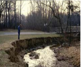
Stream bank erosion due to lack of riparian zone (buffer strip)
